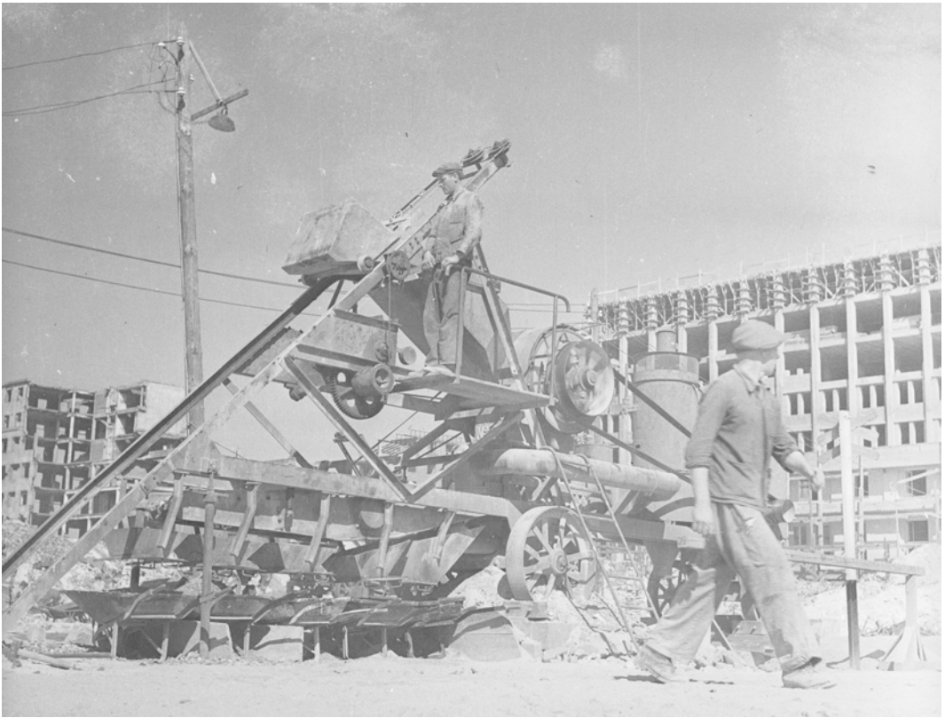
Fig. 6 - Rubble crusher and sorter in operation in central Warsaw, 1948. It is one part of the larger mechanical assembly producing air bricks, eighteen of which were acquired in Switzerland in 1946. Military Photographic Agency, National Digital Archive (WAF, 1948).
